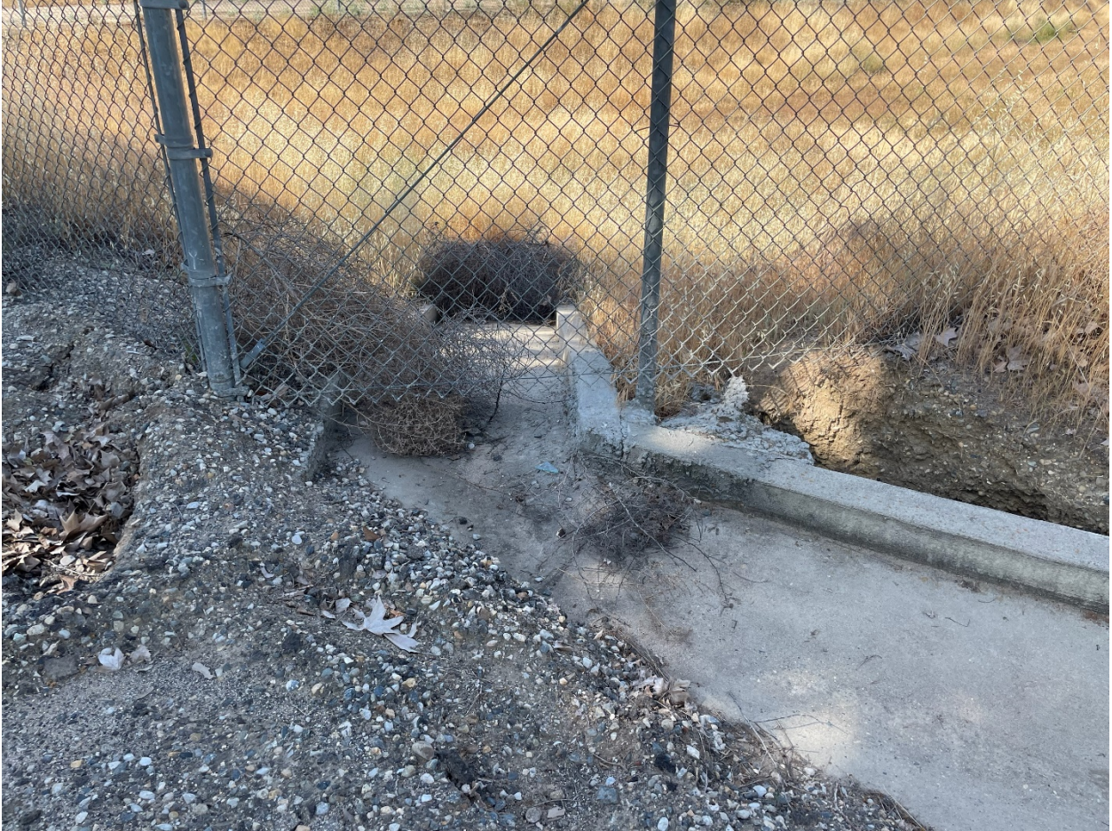
Photograph 14. Drainage Feature that connects to the Retention Basin at the 144 FW of the MCRC.
